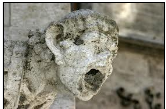
Carved stone damaged by acid rain
